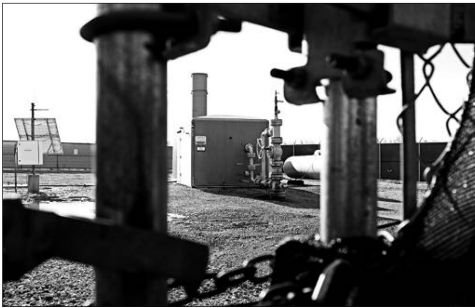
A leak in this Peoples Gas-run well tainted the water supply. State officials didn't refer the case to the attorney general's office until about 10 months after being notified of the leak.
