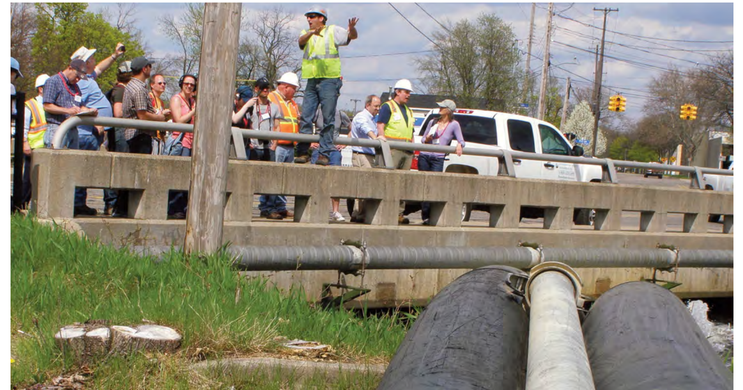
Paul Ruesch, on-scene coordinator for the U.S. EPA's "time critical" cleanup of Portage Creek, explains the logistics of rerouting the creek (through the black pipes in the foreground) so that contaminated sediment in this section of the creek in downtown Kalamazoo can be removed.
