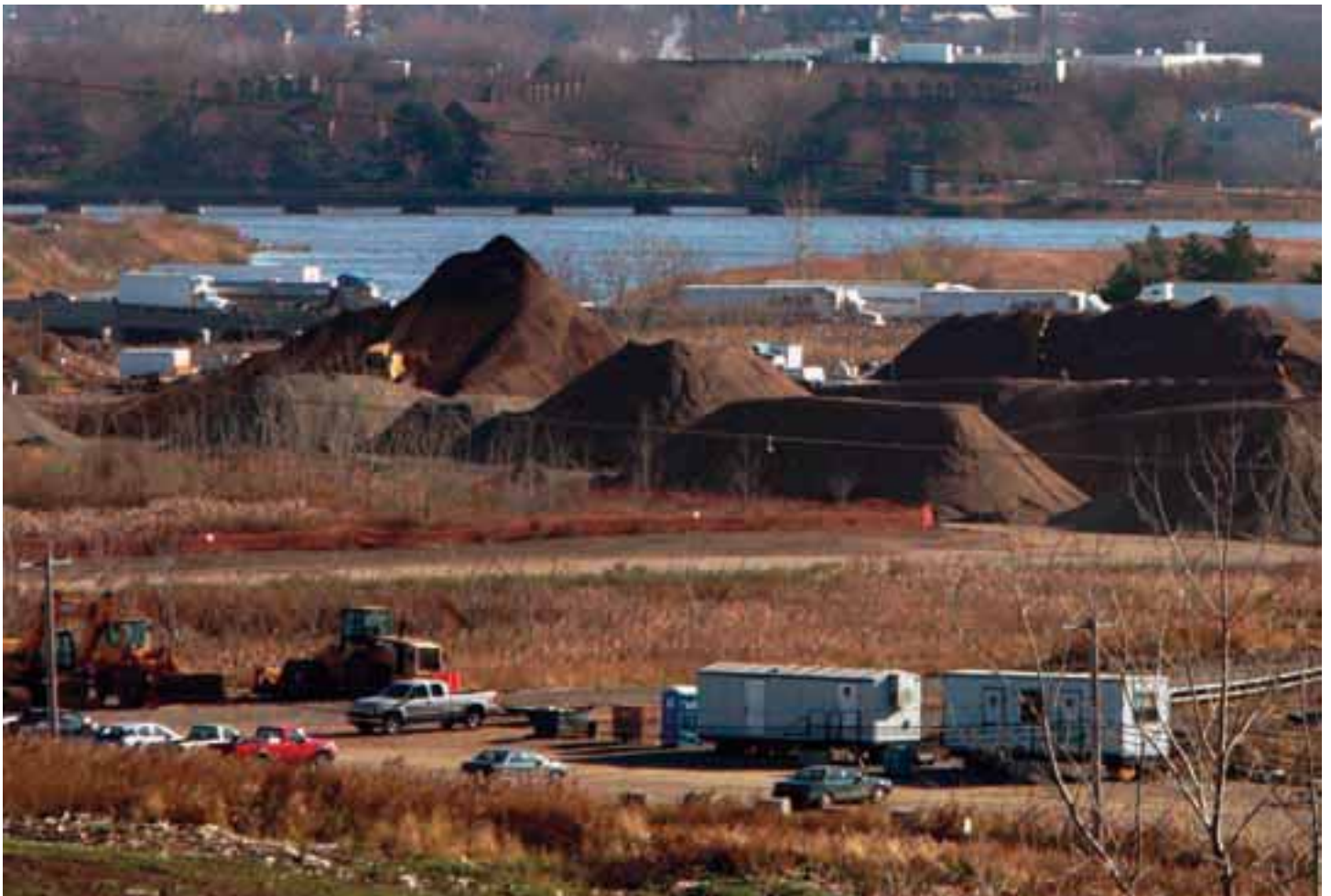
ENCAP PROJECT: The $470-million first phase of the EnCap project of creating two golf courses, nearly 3,000 housing units and a 350-room hotel on former landfills in the meadowlands in Lyndhurst and Rutherford, N.J. Photo by Thomas E. Franklin / The Bergen (NJ) Record
